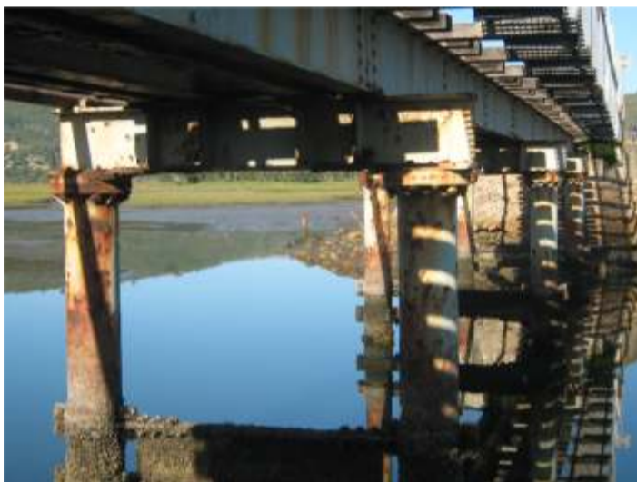
The Outeniqua Choo-Tjoe's 'Donkey Bridge' over the Knysna Estuary will need considerable repair. Image courtesy Pierre Joubert
